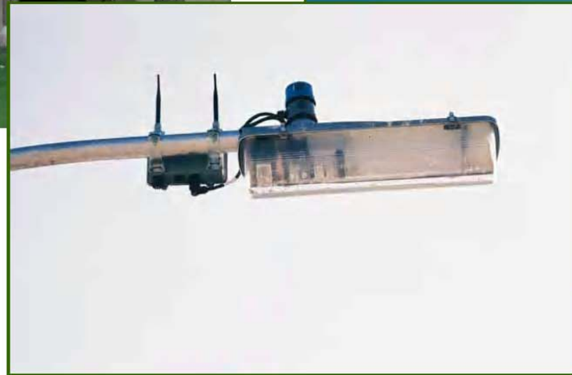
Sensoria EnRoute500 with street light power adaptor, San Diego, CA neighborhood
