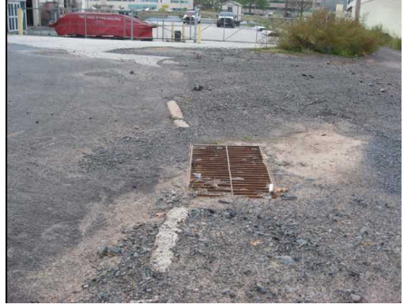
Battered storm drain – New York Drive
