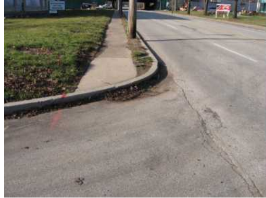
Poor sidewalk conditions – Commerce Drive
