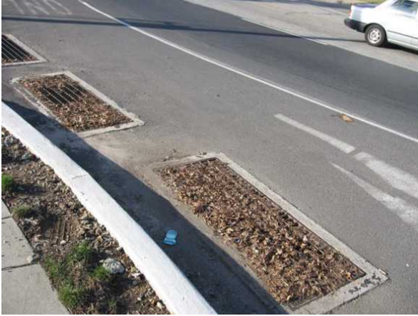
Clogged storm drains - Commerce Drive
