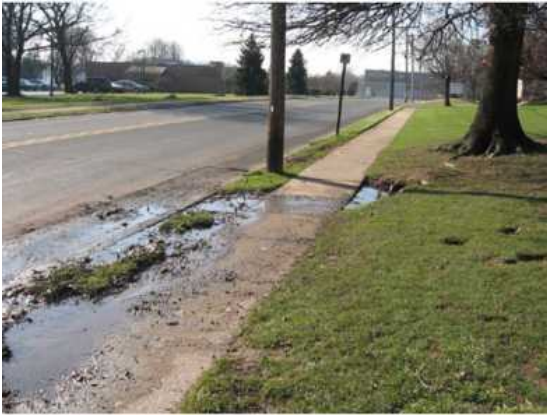
Curb failure – New York Drive
