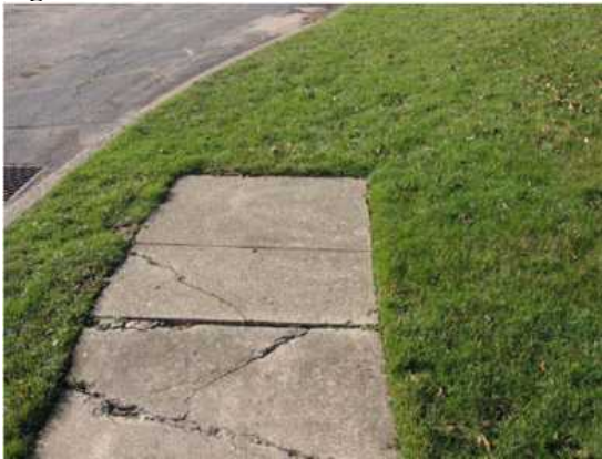
Cracked sidewalk to nowhere – New York Drive
